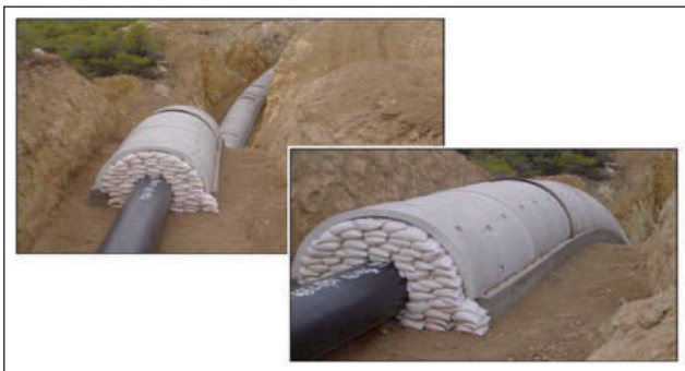
FIGURE 9 Megara to Korinthos High Pressure Natural Gas Pipeline. Encasing of pipeline at active faults crossings Source: http://users.ntua.gr/gbouck/proj-photos/megara.html
