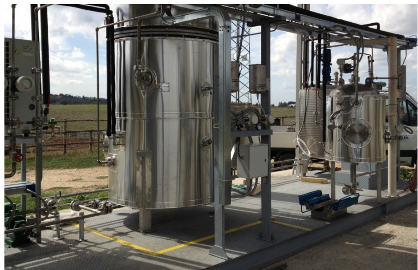
Fig. 3 Two-stage anaerobic digestion pilot plant at CREA Research Centre in Monterotondo
