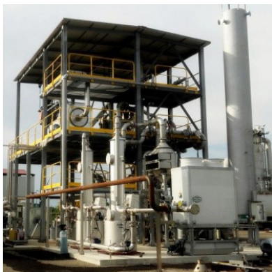
Fig. 1 Three stages gasification pilot plant
