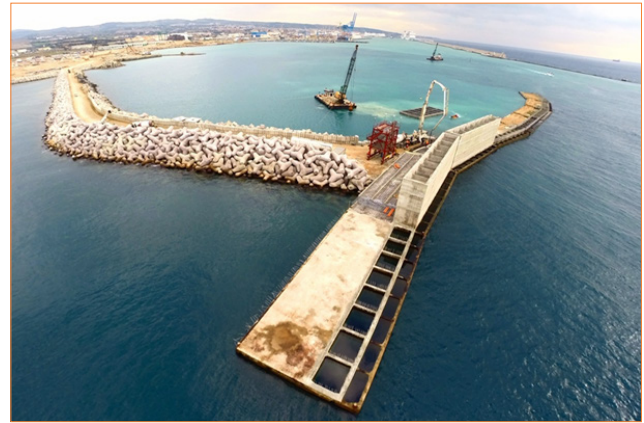
FIGURE 9 Progress of the construction of the REWEC3 caissons at the Port of Civitavecchia
