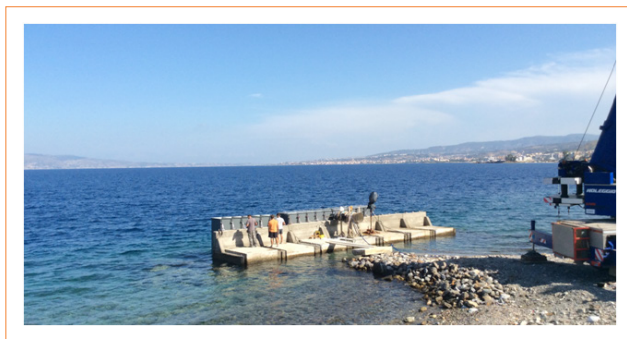
FIGURE 5 The REWEC3 caisson realized in collaboration with ENEA, during the installation stage at NOEL laboratory
