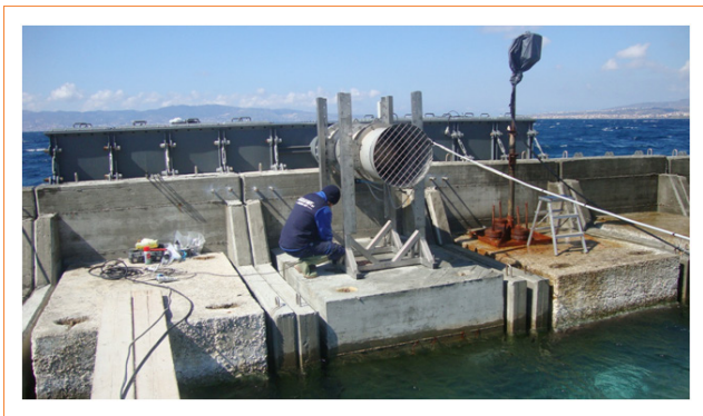
FIGURE 2 Wells turbine installed at the REWEC3 breakwater at NOEL laboratory. The turbine has been designed within the POSEIDONE project by the team of the University of Rome La Sapienza and manufactured by Faggiolati Pumps SpA. Experimental activities are managed by Mediterranea University and Wavenergy.it
