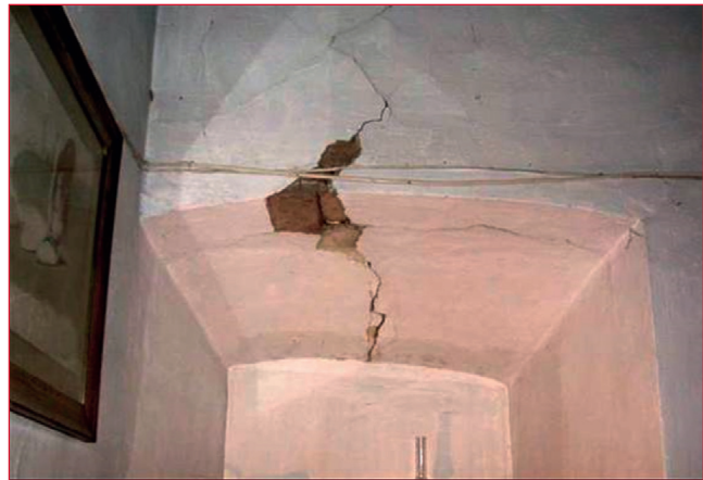
FIGURE 18 Damage to architrave
