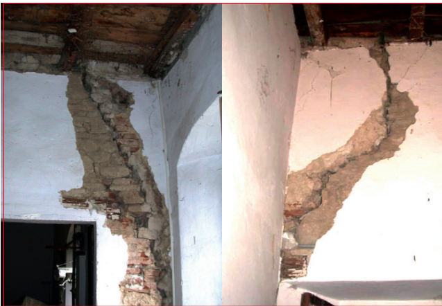
FIGURE 15,16 Cracks due to façade overturning
