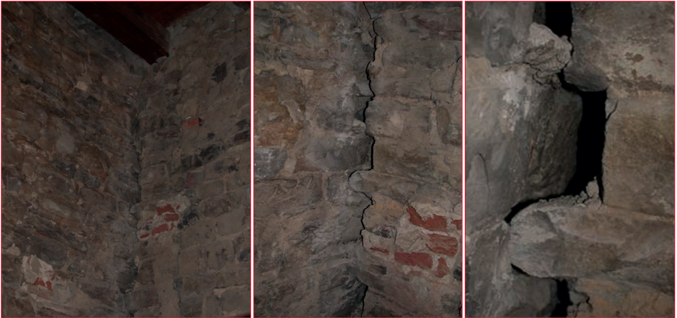
FIGURE 22,23,24 Walls detachment ascribable to 1869 Vergato earthquake
