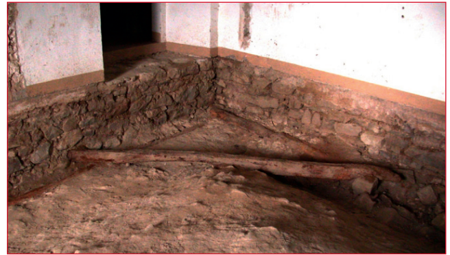
FIGURE 29 Wooden beams bending walls corner at the extrados of a pavilion vault
