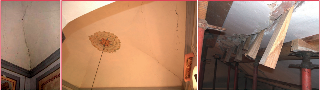
FIGURE 12,13,14 Damage to pavilion vaults
