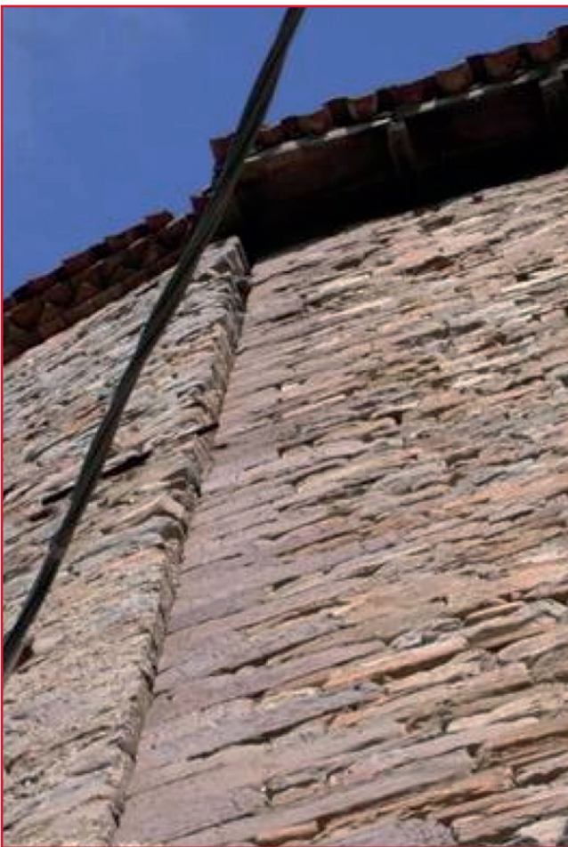
FIGURE 11 Structural discontinuity between adjacent building parts
