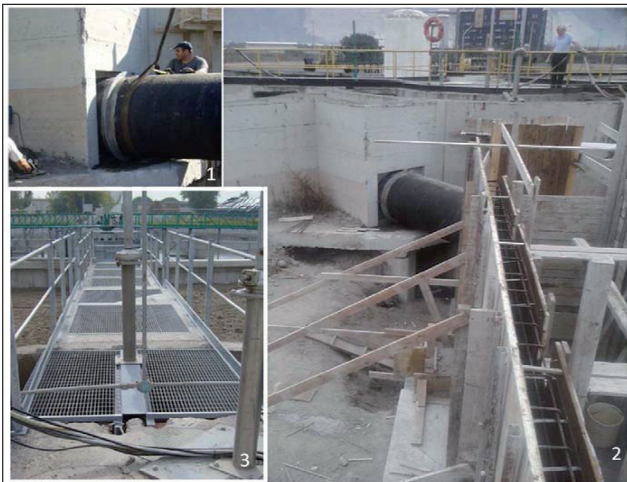
FIGURE 11 Connection of the flow splitter to the secondary clarifier (clarified water channel)
