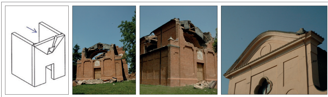
FIGURE 6 Church of S. Luca, Camurana, Medolla (photos 1&2), Church of San Francesco d’Assisi, Finale Emilia (photo 3) (drawing by [2])
