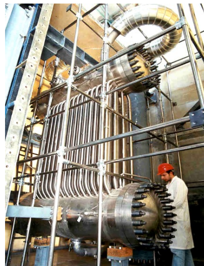
Passive Isolation Condenser
