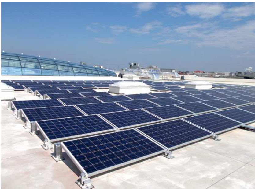
Photovoltaic system built by Conergy on the roof of the shopping center Romagna Valley Shopping in Savignano sul Rubicone
