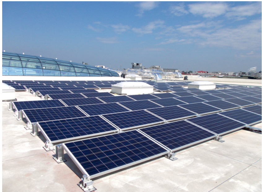
Photovoltaic system built by Conergy on the roof of the shopping center Romagna Valley Shopping in Savignano sul Rubicone
