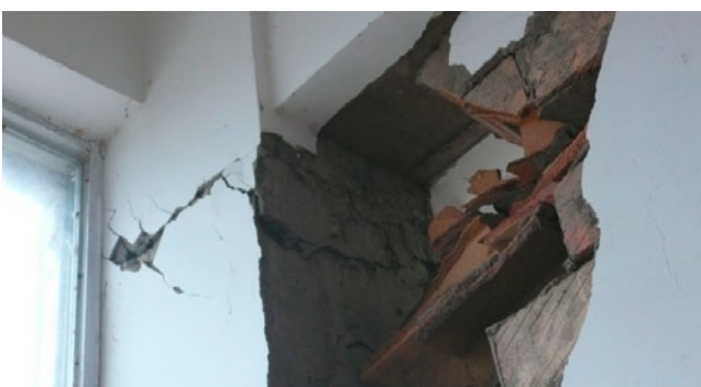
FIGURE 9 Structure damaged during the Lu Shan earthquake
