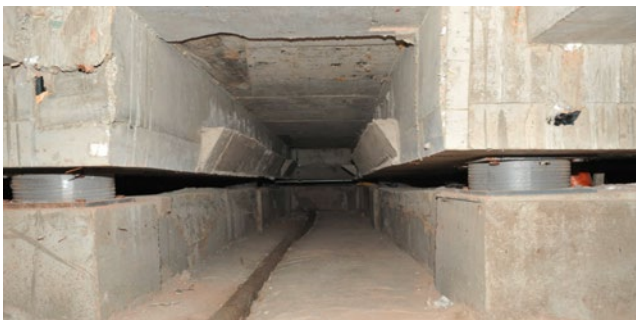
FIGURE 19 Base isolation system in a retrofitted school
