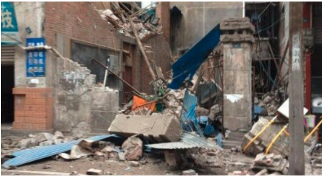
FIGURE 8 Collapse of a house building during the Lu Shan earthquake
