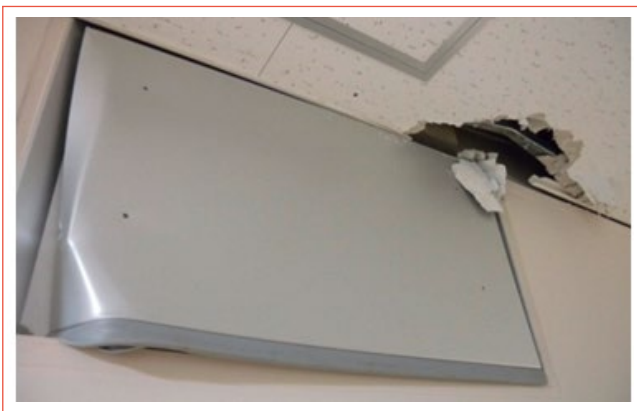
PHOTO 3 Damage to cover panel
