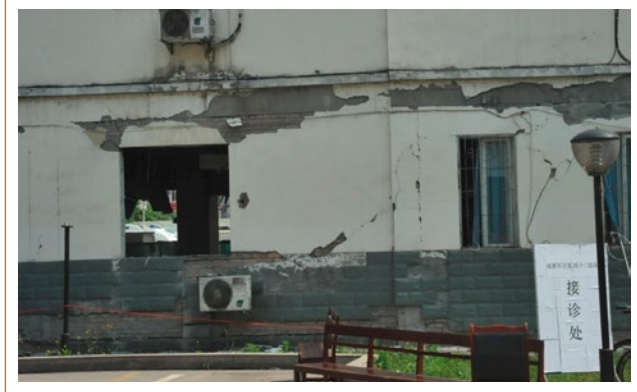
FIGURE 11 The two buildings without seismic isolation in the Lu Shan County Hospital
