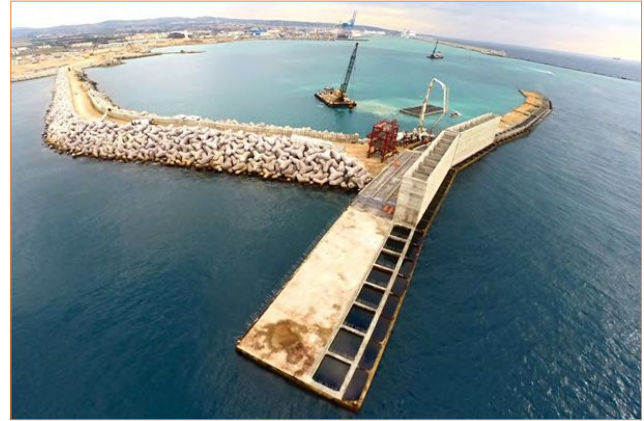
FIGURE 9 Progress of the construction of the REWEC3 caissons at the Port of Civitavecchia
