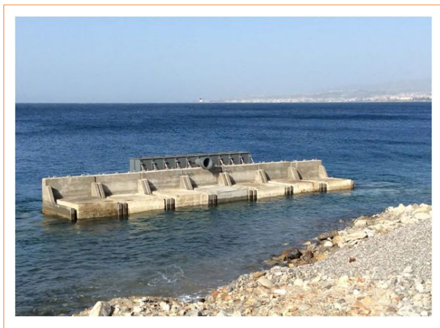
FIGURE 1 The REWEC3 plant installed in the breakwater in reinforce concrete at NOEL laboratory
