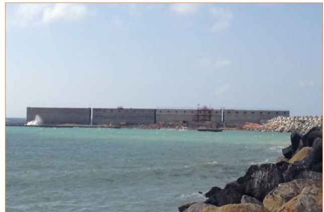
FIGURE 10 4 REWEC3 caissons completed up to 10m above M.W.L. at the Port of Civitavecchia (Rome, Italy)
