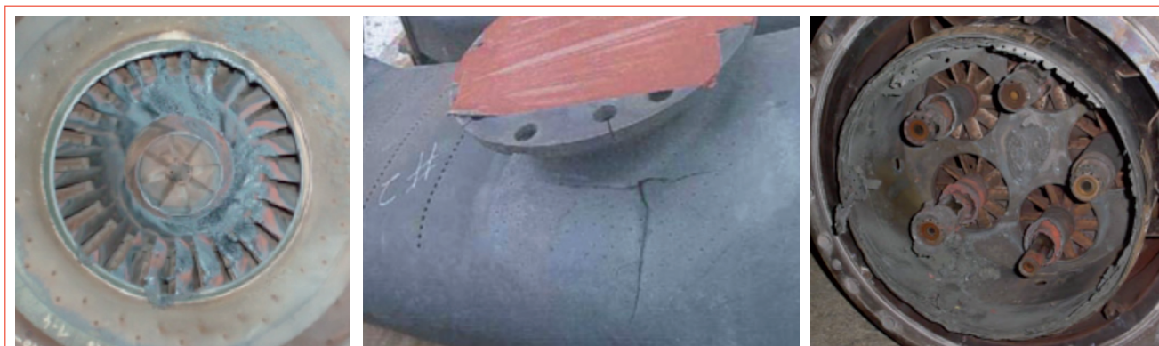
FIGURA 2 Examples of damage. (a) Burner damage caused by flashback due to high levels of higher hydrocarbons 8 . If proposals to store / transport energy by adding hydrogen to the natural gas transmission system are implemented, the potential for flashback is likely to increase on some burners. (b) Cracks due to low-frequency (150 Hz) thermo-acoustic instabilities. (c) Damage due to high-frequency (2350 Hz) thermo-acoustic instabilities, in this case due to inappropriate tuning of the machine 9
