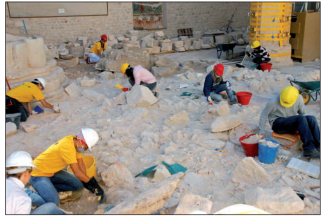
FIGURE 6 Restoration and screening of the ruins in the Church of S. Maria di Collemaggio in L'Aquila, following the 2009 earthquake Source: Author's personal archive
