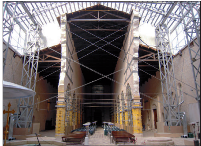
FIGURE 7 Securing and roofing the transept in the Church of S. Maria di Collemaggio in L’Aquila, following the 2009 earthquake
