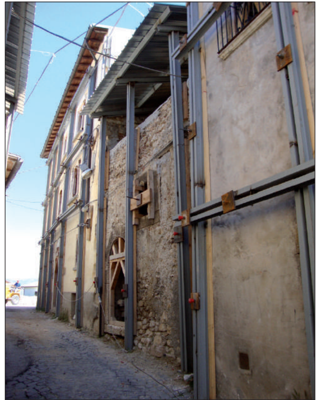
FIGURE 12 Securing historical palaces in the historical centre of L'Aquila, following the 2009 earthquake Source: Author's personal archive
