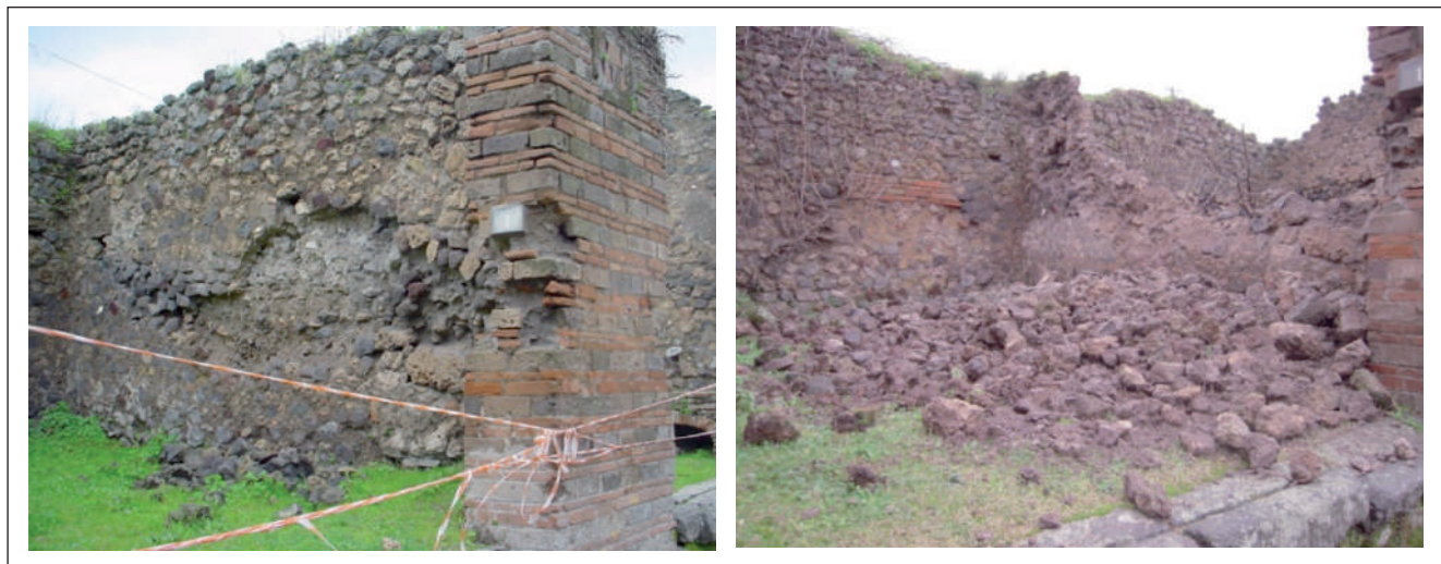
FIGURE 1 Wall in Regio VII (Insula 2, No. 1), (a) before and (b) after the collapse Source: Soprintendenza Speciale per i Beni Archeologici di Napoli e Pompei
