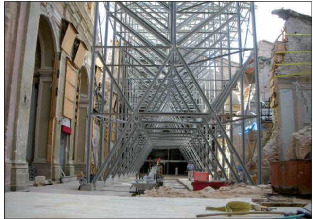
FIGURE 9 Securing and roofing the Church of S. Maria di Paganica in L'Aquila, following the 2009 earthquake Source: Author's personal archive
