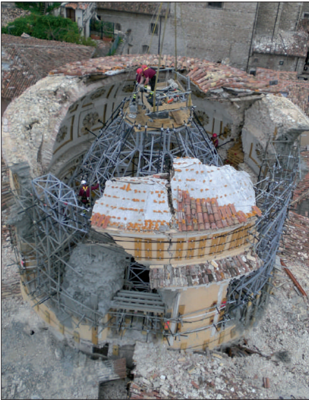
FIGURE 8 Securing the dome of the Church of S. Maria del Suffragio in L'Aquila, following the 2009 earthquake Source: Author's personal archive
