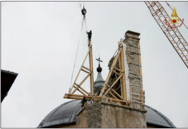
FIGURE 5 Securing the bell gable of the Basilica di S. Bernardino in L'Aquila, following the 2009 earthquake Source: Author's personal archive
