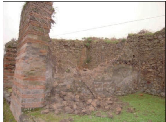
FIGURE 5 Walls showing different structural behaviors and resultant damage Source: Soprintendenza Speciale per i Beni Archeologici di Napoli e Pompei
