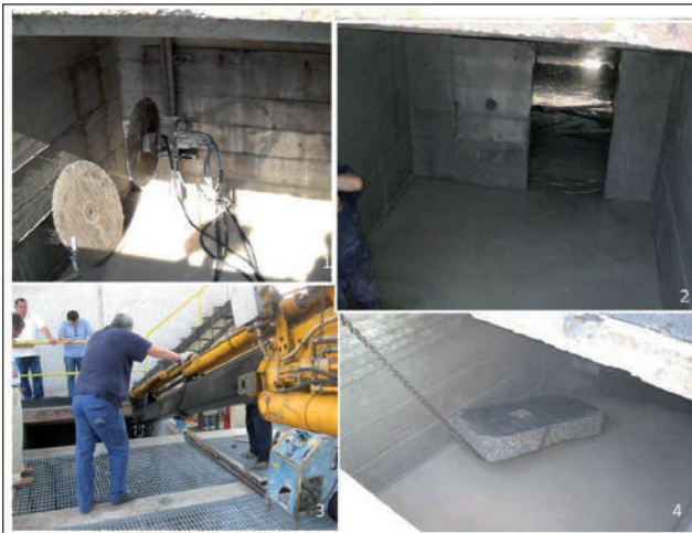
FIGURE 9 Connection sequence for junction of feeding flow splitter chamber and new biological basin
