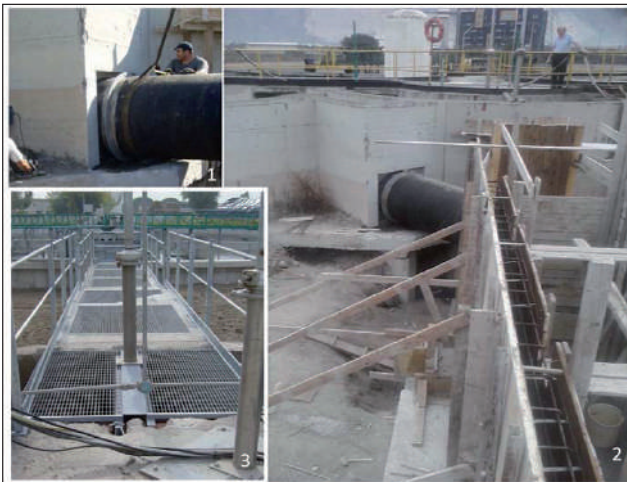
FIGURE 11 Connection of the flow splitter to the secondary clarifier (clarified water channel)
